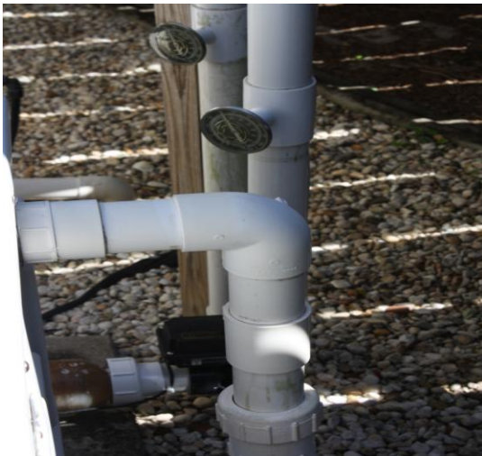
Figure 5 - Solar Pool Heat Controls
