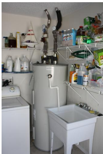
Figure 3 - Solar DHW storage tank, pump, control valves, thermometers
