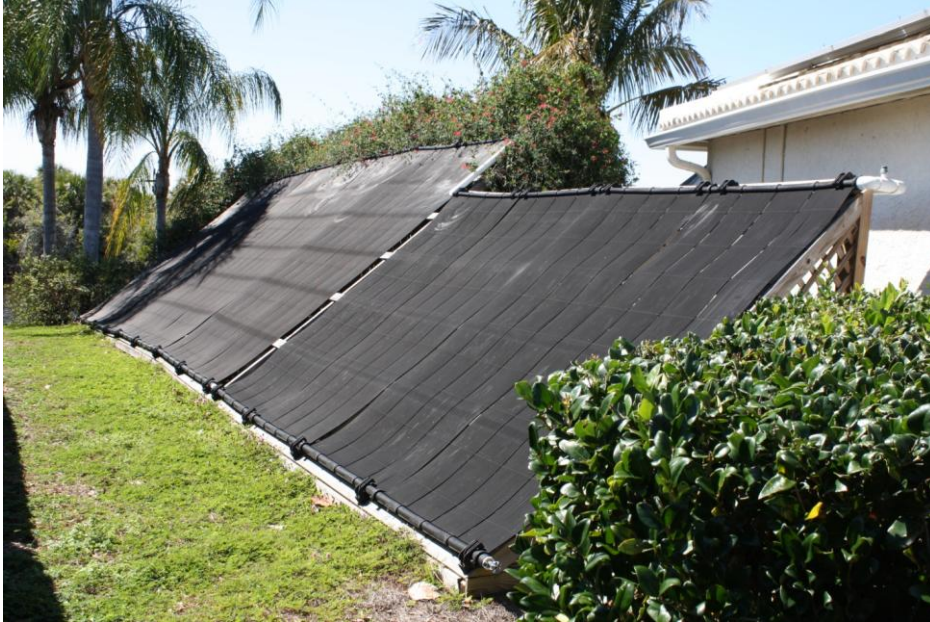
Figure 4- Solar Array Pool Heat
