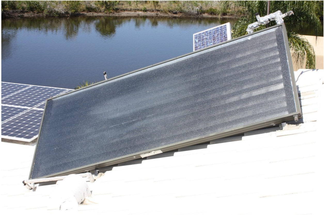
Figure 2- DHW Collector with PV module to run pump
