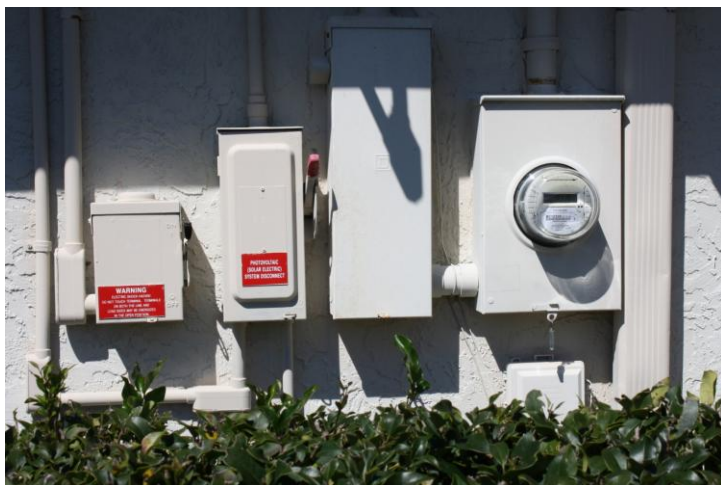
Figure 9 - Meter and Junction Boxes
